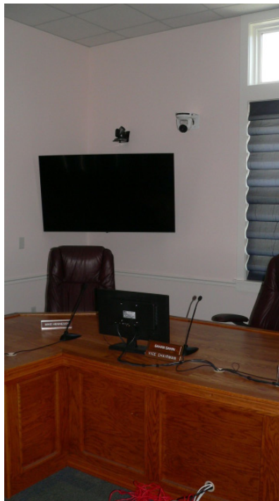
New camera (top right) installed in Arcand Meeting Room
