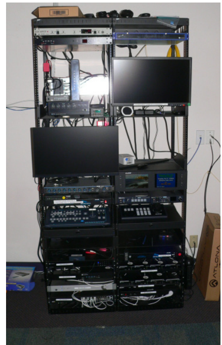
Upgraded video closet at the Bellingham Town Hall
